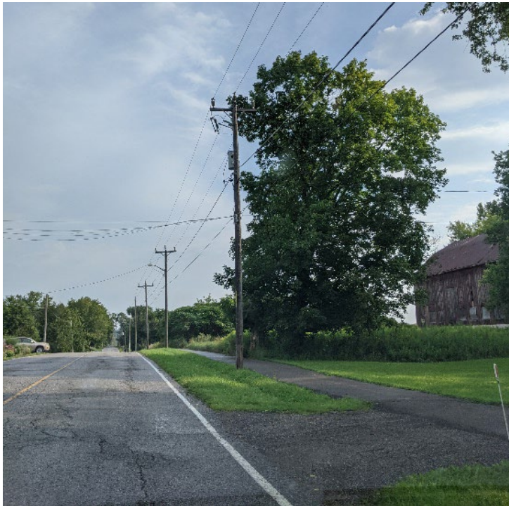
Photo 1 – View of off-site pole-mounted transformer west of barn, facing north.
